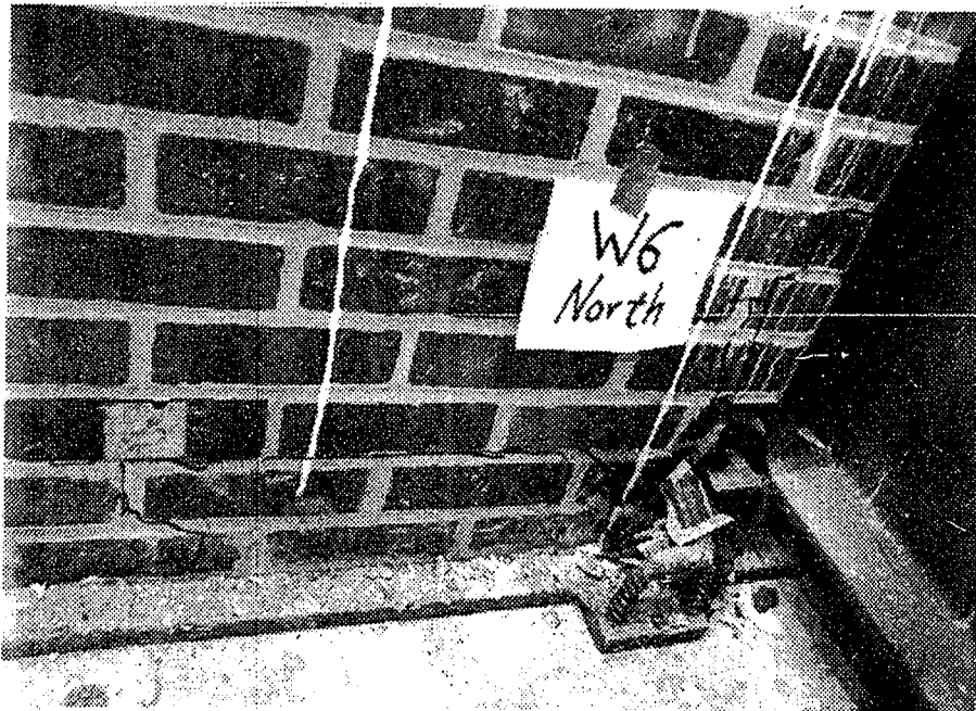
b) Bearing failure in wall "W6"
